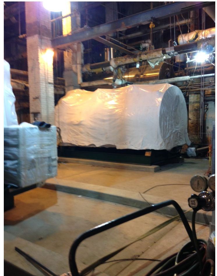
New Boilers in Plant
